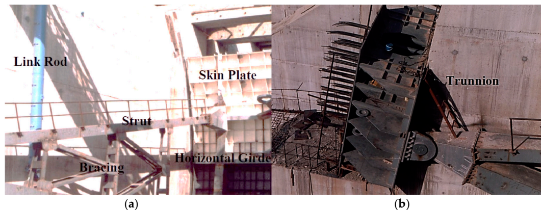
Figure 2. Primary radial gate components of Karkheh Dam (a) truss and skin plate, (b) trunnion beam.
