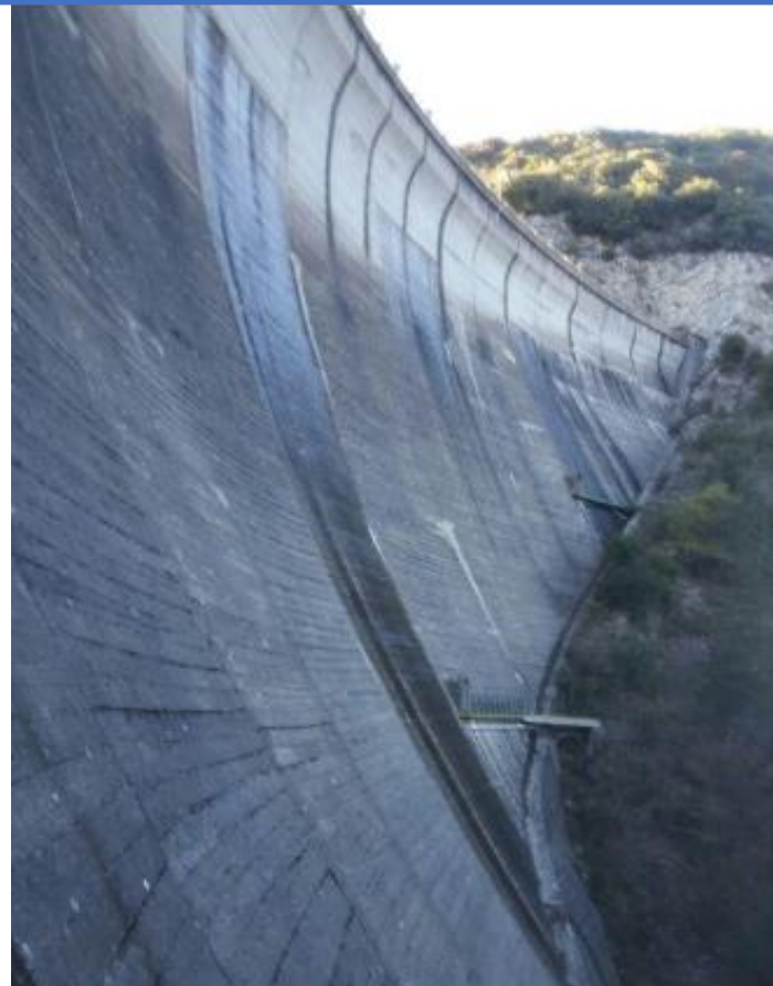
Fiastrone Dam. Increased seepages on the downstream face after 30th Oct 6.5 Mw earthquake.
